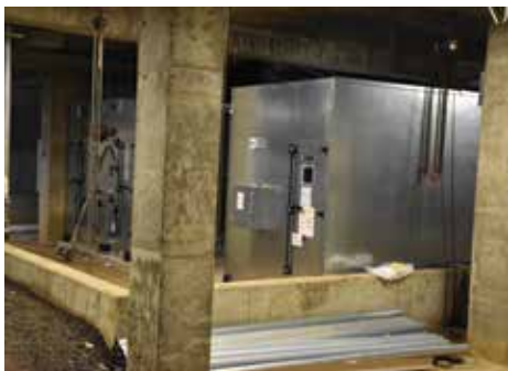
New HVAC systems will dramatically improve comfort, air quality and efficiency for students and staff at CNS High School.
